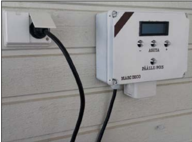
Figure 10. A fully assembled and functioning system in the real world.
